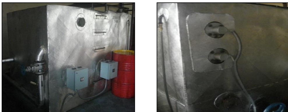
Gambar 7. Service tank MFO.
