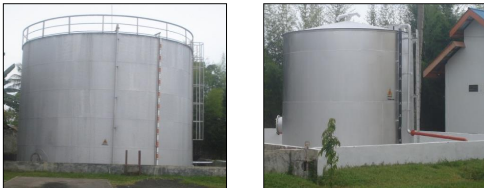
Gambar 6. Storage tank MFO dan HSD.
